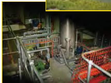
Duplex priming system and priming tank
